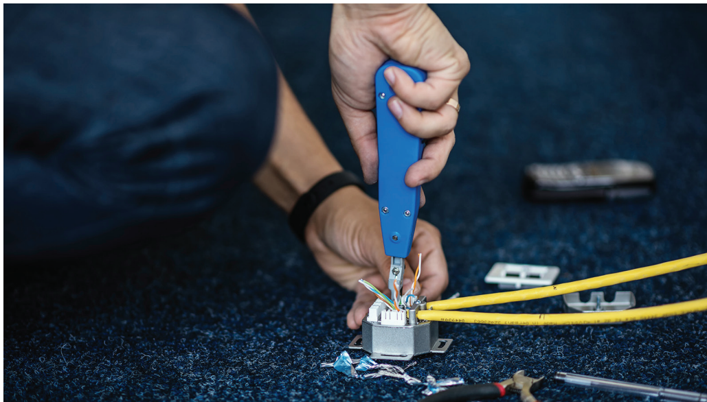
Adding RJ-45 terminals to a network cable using a punchdown tool. (Image by dero2084 © 123RF.com.)
