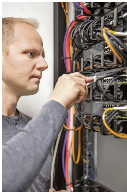
Verifying patch cord connections. (Image by Kjetil Kolbjornsrud © 123RF.com.)
