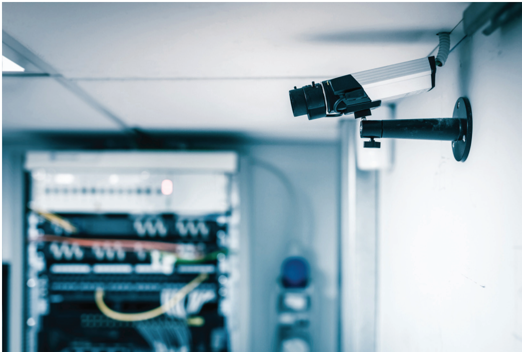
Pan-tilt-zoom CCTV installed to monitor a server room. (Image by Dario Lo Presti © 123RF.com.)
